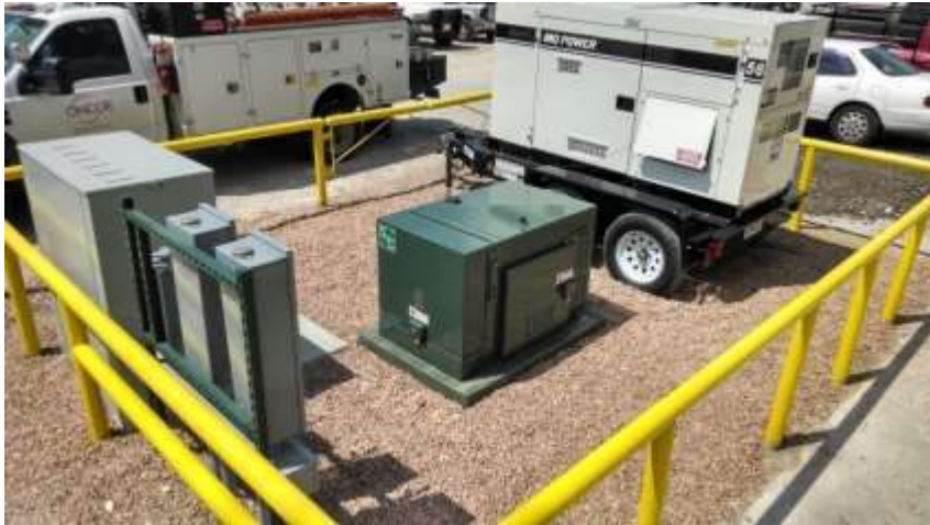
Oncor Initial Installation at Oncor Facility
