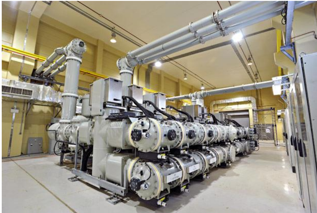
Gambar 2 : Gas Insulated Substation (GIS)
