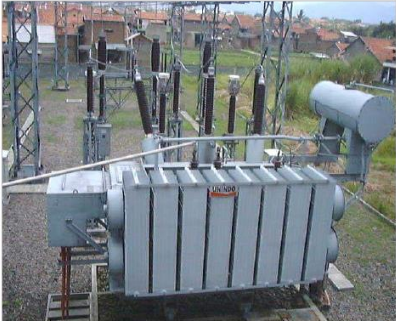
TRANSFORMATOR TENAGA 150/20 kV 30 MVA
