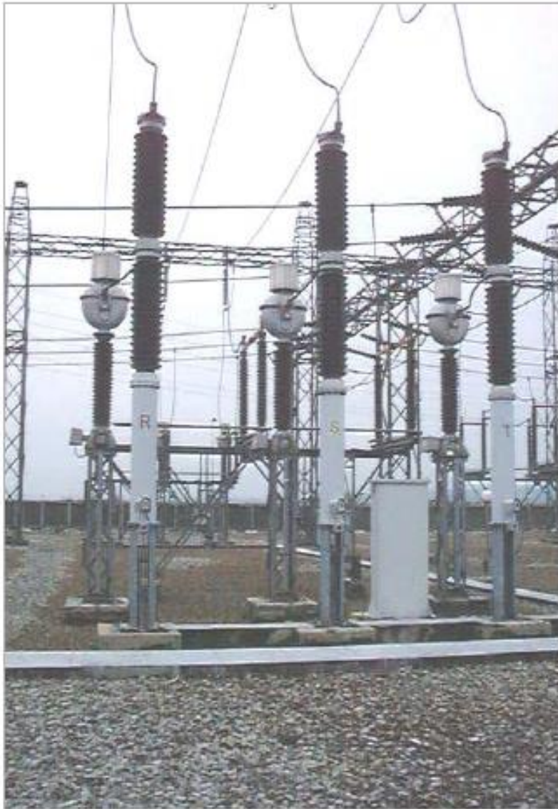
LIGHTNING ARRESTER 150 kV
